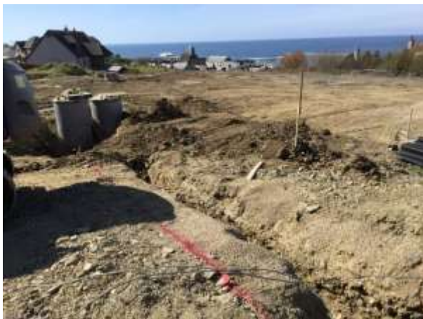
Clearing of site to allow for suitable ground conditions and house foundations – typical sunny day in MacDuff.
