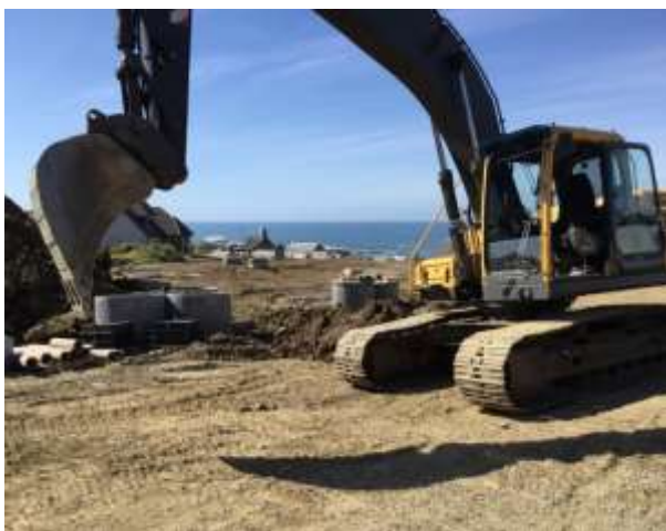
Digger on site to dig drainage and sewerage routes through the site
